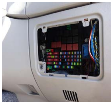
Figure 7-2.2 Inside View - Electrical Junction Box Location
