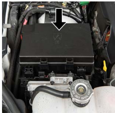
Power Distribution Center
