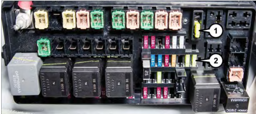
Power Outlet Fuses
