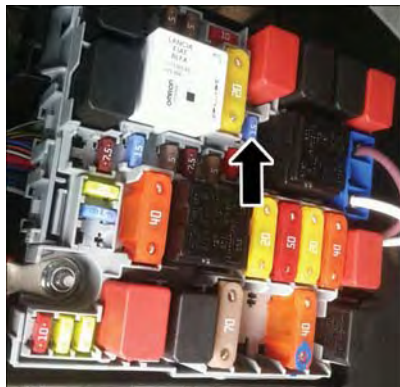
Power Outlet Fuse Location
