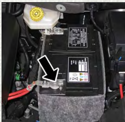
Positive Battery Post
