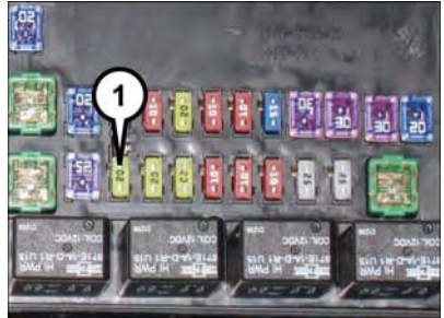
Rear Quarter Power Outlet Fuse
