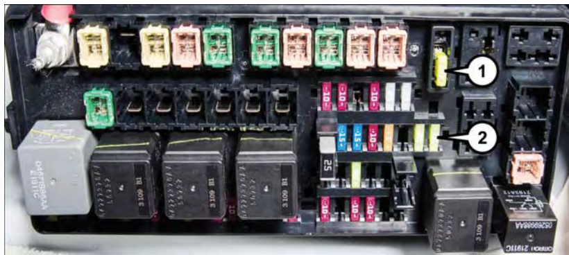
Power Outlet Fuses
