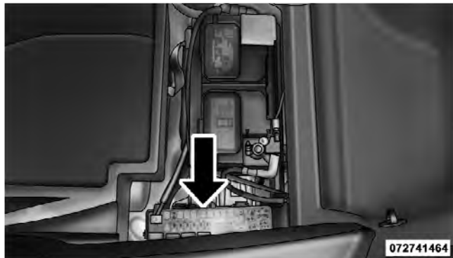
Rear Power Distribution Center
