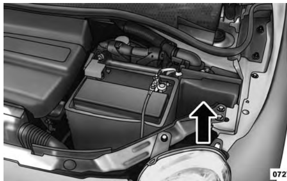
Front Distribution Unit
